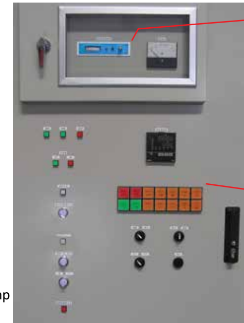
Interface and Water Cooling Panel
